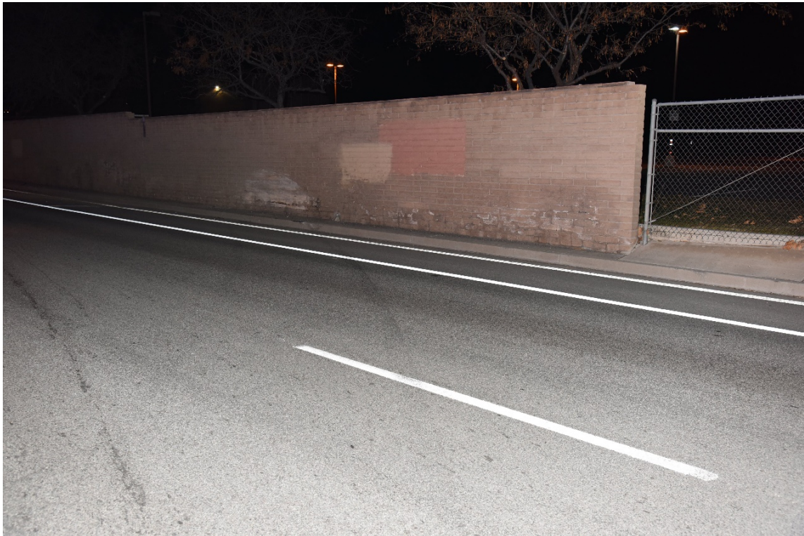
The brick wall on the north side of McCarran where Lee crashed.
